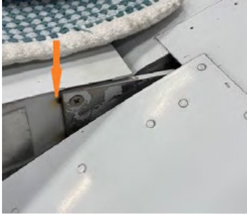
Photo: AA5 Nutplate Corrosion.jpeg
